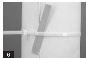
6. Larger diameter columns require joining two straps together. Temporary shims maybe required to align the column seam. The shims are removed after the polyurethane adhesive has cured
