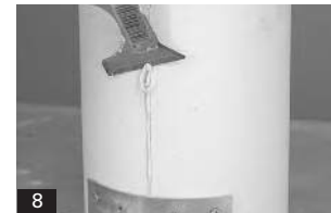
8. Allow the polyurethane adhesive to thoroughly cure and cut away the straps. Use a putty knife to remove any excess polyurethane adhesive. Use automotive body filler to cover any voids along each seam. Sand both seams smooth.
