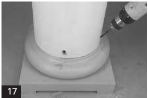
17. Pre-drill and countersink holes at an angle through the shaft into the base wood plug. Install rust resistant screws to secure the shaft to the base wood plug. Remove any excess paintable silicone sealant.
