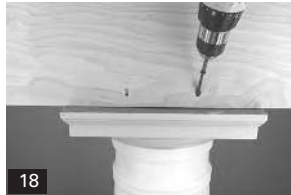
18. Pre-drill and countersink holes at an angle through the soffit into the capital wood plug.
