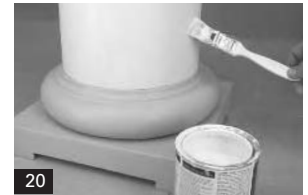
20. Finish the column by applying a final coat of exterior oil-based paint.
